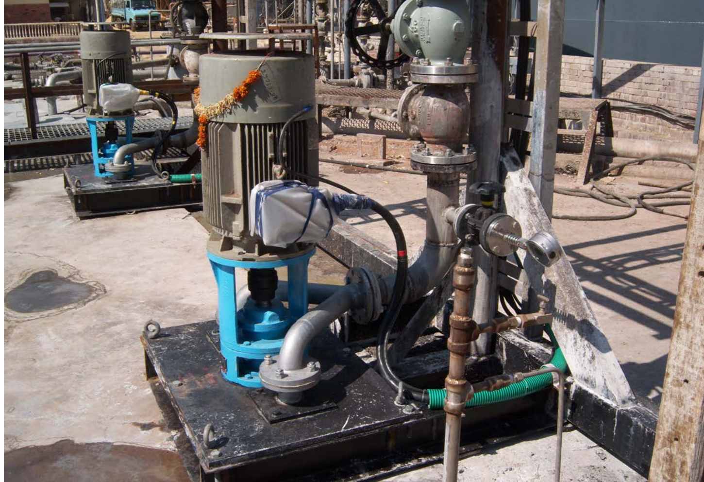
KISHOR make Vertical (VS4) pumps in parallel at a fertilizer plant in Goa
