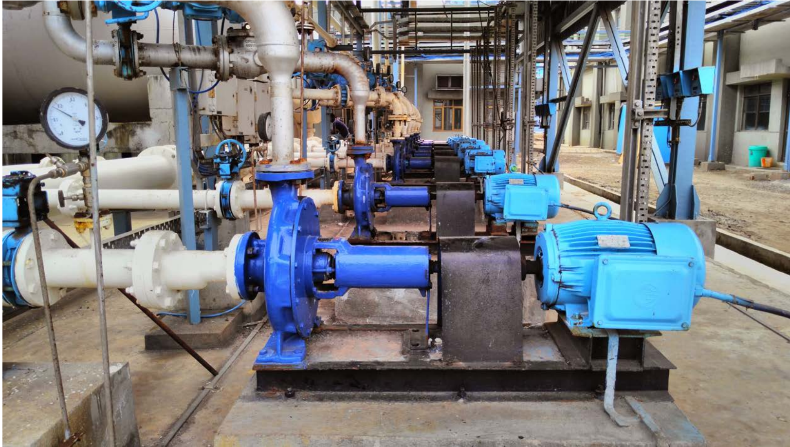
KISHOR make Horizontal end suction pumps in parallel at a desalination plant near Chennai
