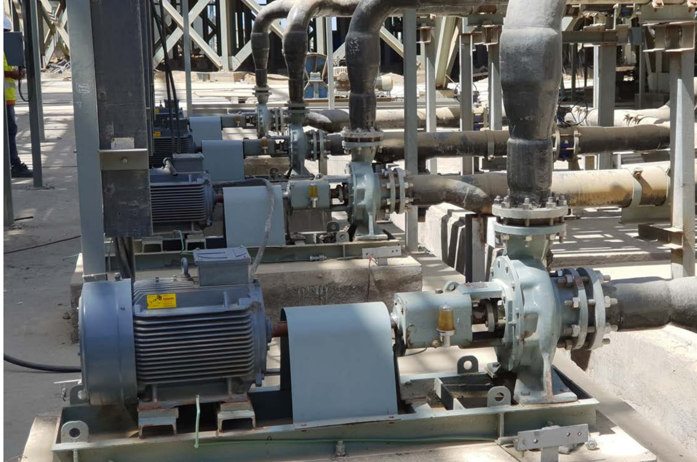
KISHOR make Horizontal end suction pumps in parallel at a soda ash plant in Gujarat
