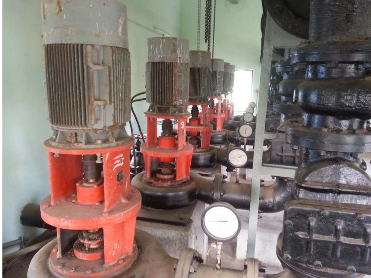
KISHOR make Vertical Dry Pit Non-Clog pumps in parallel at a sewage pumping station in Vijayawada
