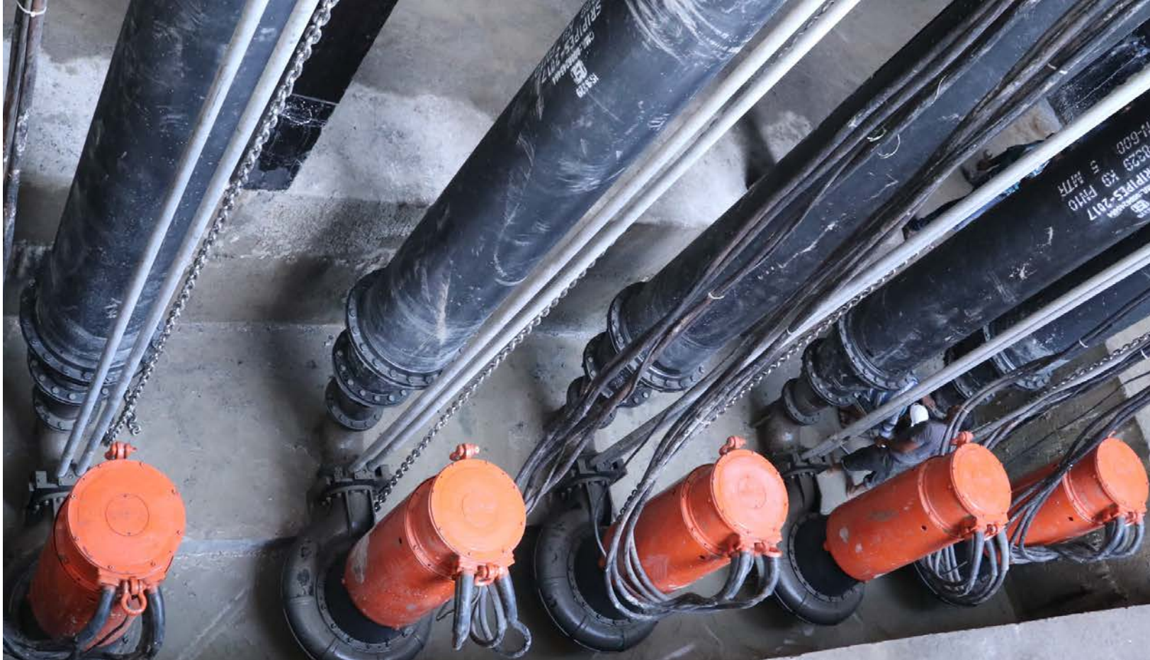
KISHOR make submersible non-clog wet pumps in parallel at a sewage treatment plant in Aurangabad, Maharashtra
